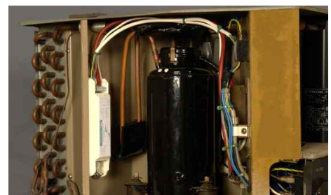
10 Check correct wiring & replace covers
