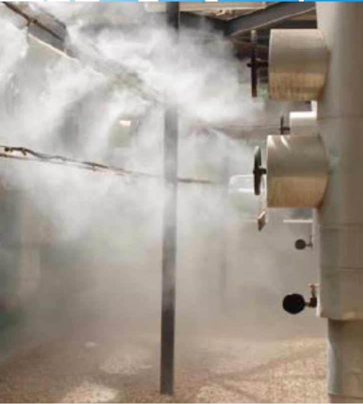
Fog nozzles placed in front of condenser coils reduce heat, save energy
