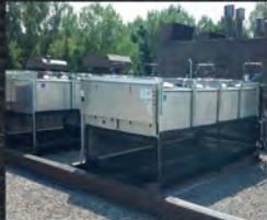
Grocery Store Chain Rooftop Condensing Units
