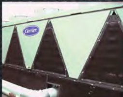
Electronics Manufacturing Plant Condensing unit with Microchannel Coils
