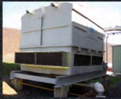
Osram, Sylvania Plant Thermal Care Cooling Tower
