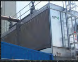
Glass Processing Plant Cooling Towers
