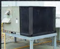
Physios Laboratories HVACR Equipment
