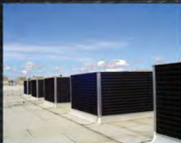
Office Building Rooftop Economizers
