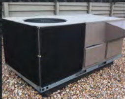
Office Building Rooftop AC Unit
