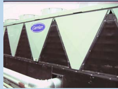
Custom-shaped triangle filters ensure optimum efficiency and simplify maintenance on this Carrier micro-channel coil laboratory cooling equipment in Plano, Texas.
