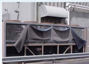
A York chiller with ineffective, disposable filters.
